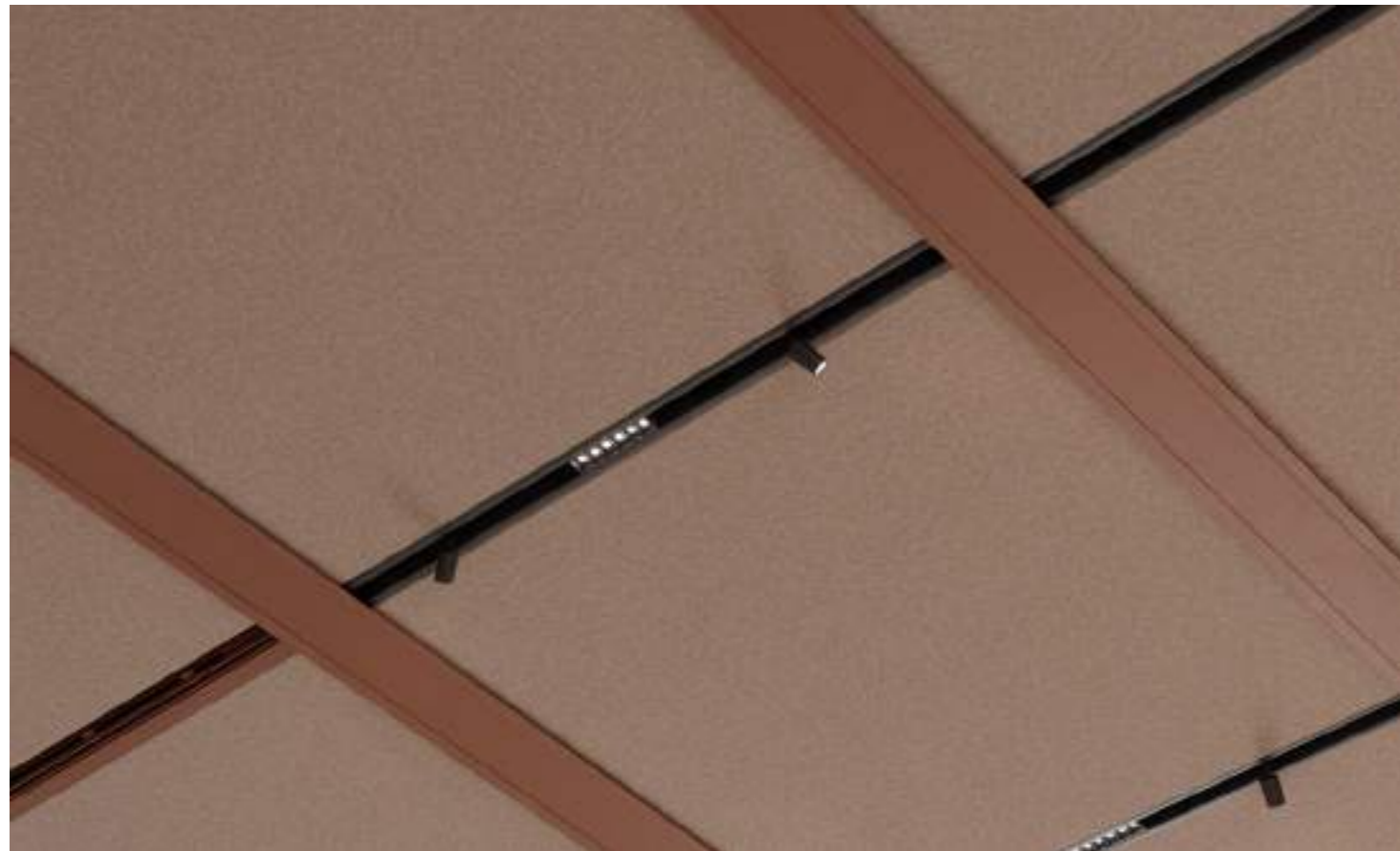
Room Flow air conditioning
